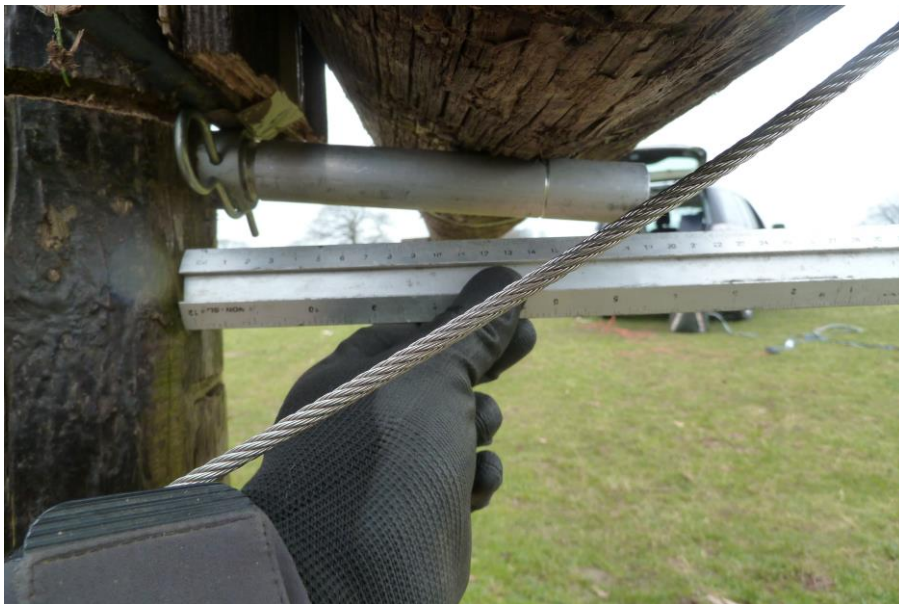
Figure 7 – A pin indicating fatigue by bending which is clearly visible
